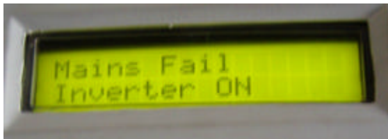
Mains Power OFF (Power Failure)
