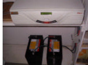
using a 24V/102Ah Battery Bank
