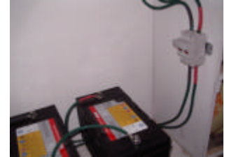
and twin 40A fused Battery Isolator
